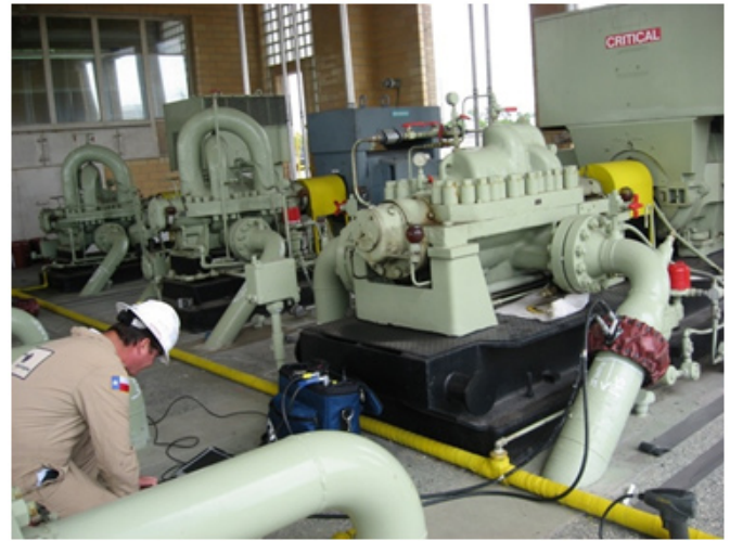
Difficult pipe inspection of pipe through concrete in the pump station
