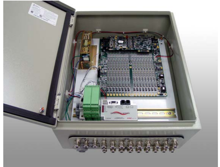
Figure 1. Inside the Sensor Highway Cabinet
