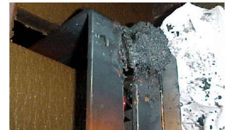
Overheated bus bar with carbon build-up
