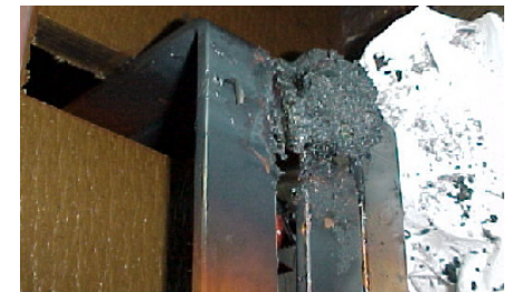
Overheated bus bar with carbon build-up
