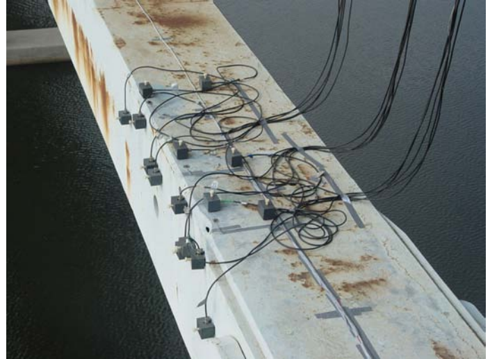
Figure A1: Box beam instrumented for AE monitoring.
