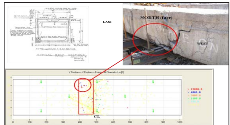
Figure G1: Location of AE events shows rupturing of prestressing strand.
