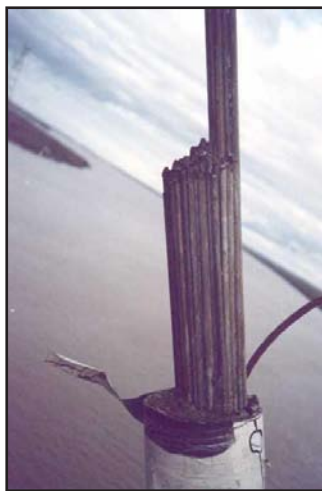
Figure D3: Failure site of cable-stay support - note multiple strand failures.
