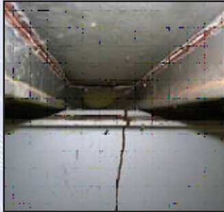
Deep stringer crack from defective weld detail in steel bridges
