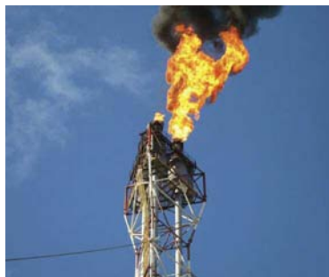
Figure 1. Primarily safety devices, flare systems collect and route waste gases (released through pressure relief valves or leaked from plant equipment) through piping runs called flare headers to elevated flare stacks, where they can be burned under controlled conditions.
