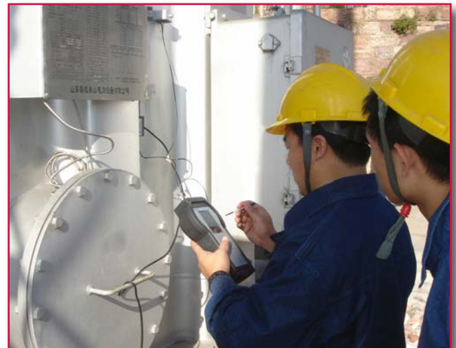
On-site real time partial discharge screening test with a Pocket AE-Power.
